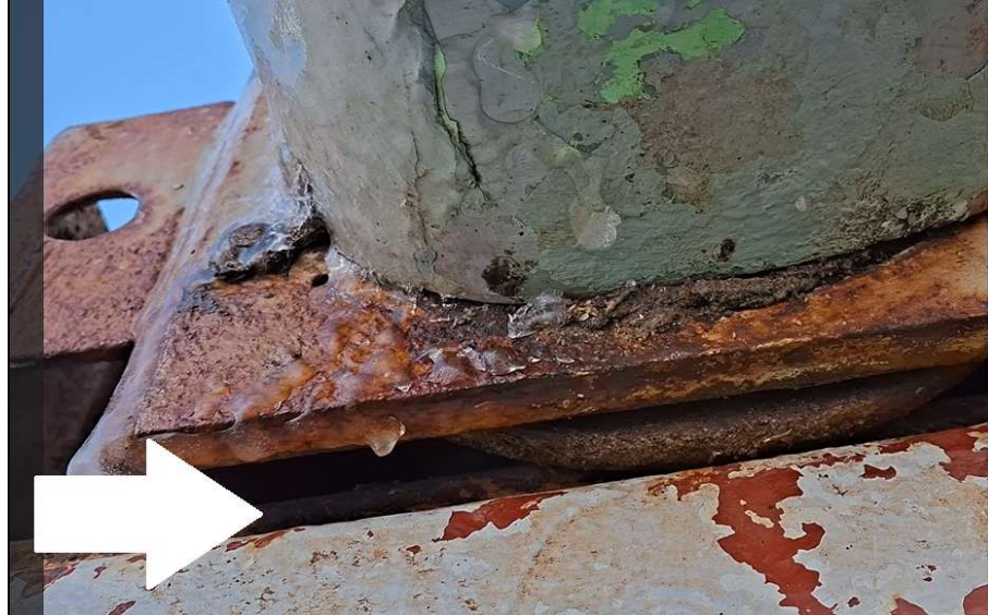
Image5. Location of nipped leg at wheeling mechanism of the crane
